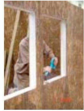
Preparing a panel installing a panel cutting an opening preparing a window
